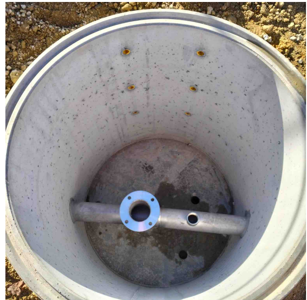
Cliff Road Pump Station – Internal stainless-steel fabrication to accommodate pump over assembly & chemical injection
