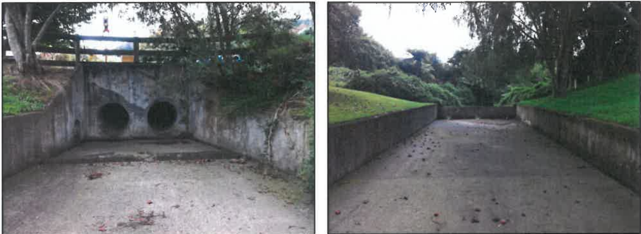
Figure 3-4: Walford Drive energy dissipation structure inlet (left) and outlet (right)
