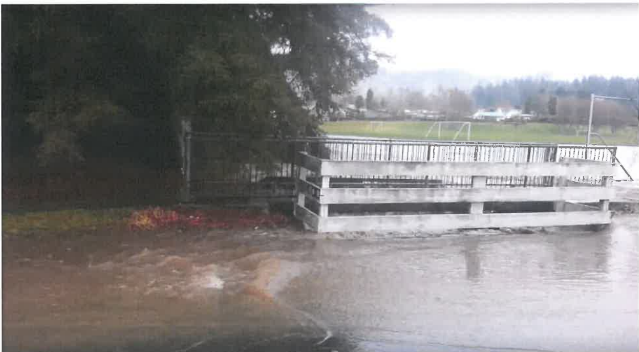
Figure 8-2: Still image from video of Te Ngae Road flooding, August 2014. Western drainage system showing the culvert inlet screen potentially overloaded and view of flooding extent in Neil Hunt Park.
