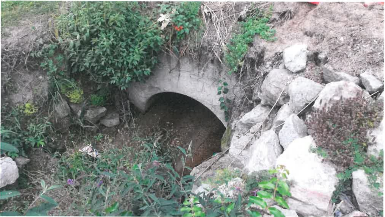
Figure 3-2 – Downstream face of Selwyn Road Culvert showing significant siltation and reduction in available cross sectional area.
