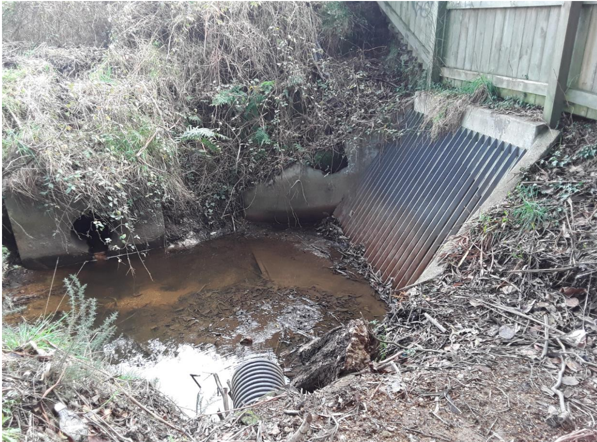
Figure 9: Trash screen for 1200mm culvert from Boielle Park
