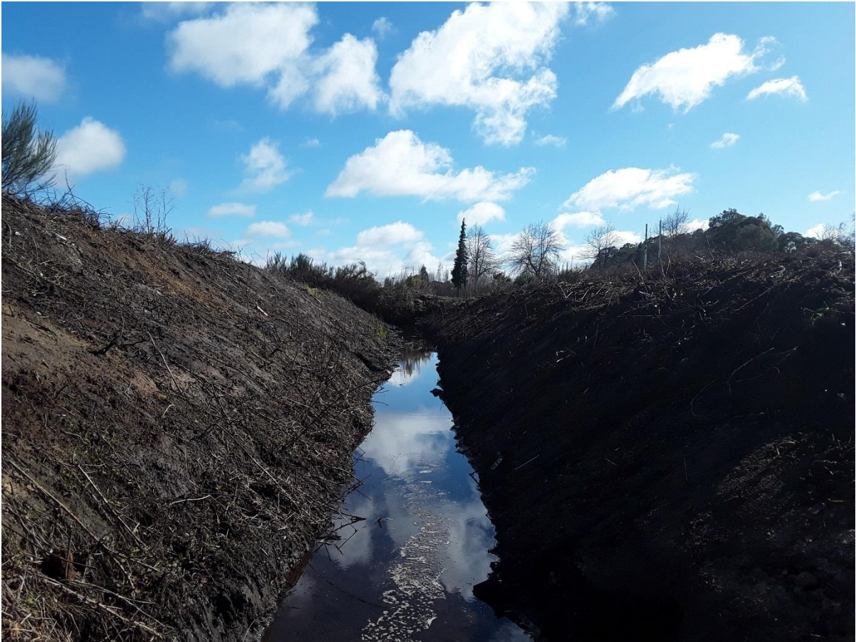
Figure 7: Drain DN004268/Xtra02 after clearing of blackberry
