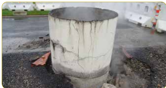
Figure 5 Bore Casing Failure (photo: Rotorua Lakes Council).
