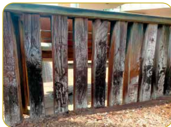
Figure 17 Timber affected by geothermal conditions (photo: (Kim Smith, January 2024).
