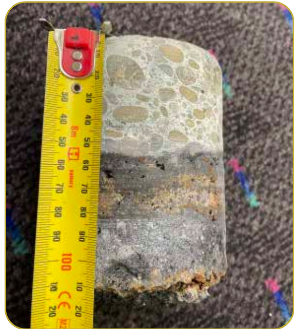
Figure 7 Concrete core showing effects of geothermal corrosion (Photo: Ash Bowtell)
