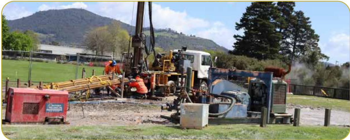
Figure 22 Example of space required around a bore for a drilling rig and plant (photo: Rotorua Well Drillers).
