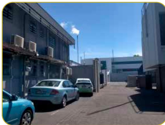
Figure 21 Geothermal venting structure (photo: Kim Smith, January 2024).
