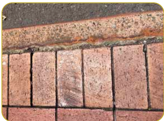
Figure 16 Concrete edging at ground level affected by geothermal conditions (photo: Kim Smith, January 2024).
