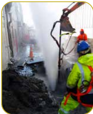
Figure 4 Bore Failure, 2016 (photo: Andrew Austin).
