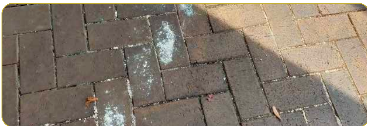
Figure 18 Deposit of salts on paving (photo: Kim Smith, January 2024).
