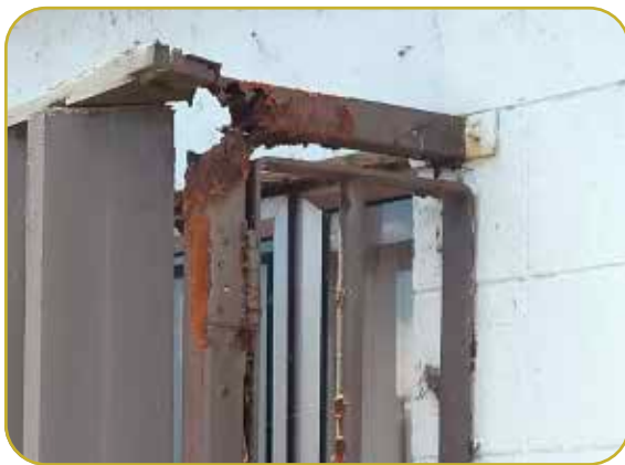
Figure 8 Accelerated corrosion on a building near Sulphur Bay (Photo: Kim Smith, January 2024).
