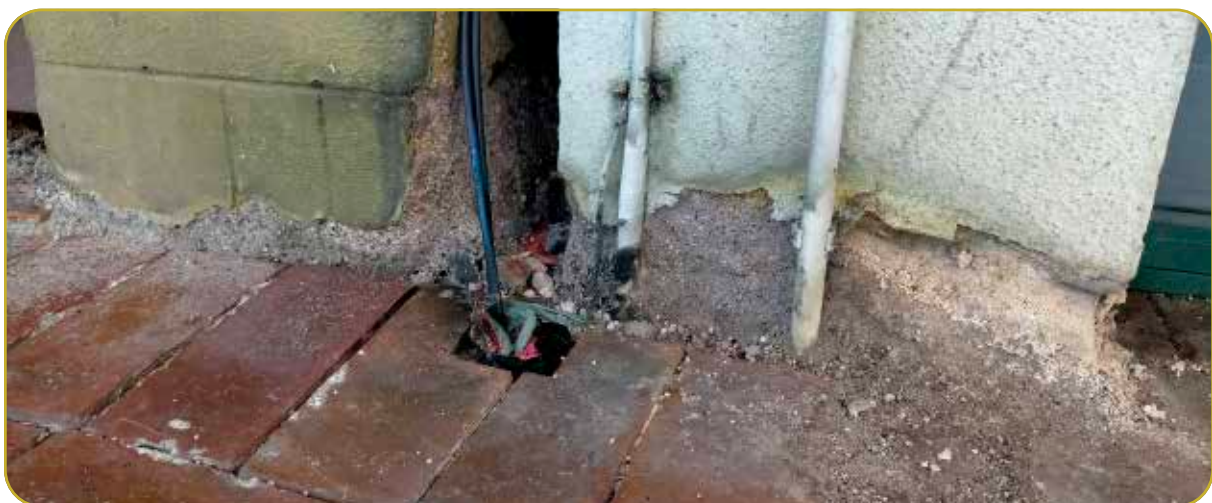
Figure 24 Deterioration of building materials at ground level (photo: Kim Smith, January 2024).
