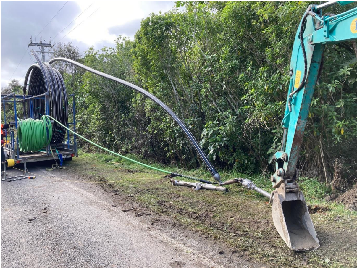
Pipe Attached to the drill head ready to be pulled through the pre-drilled hole
