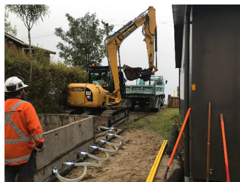
Installation occurring along Tamatea St within the confines of a tight driveway
