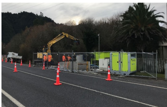
Installation of alternative flow meters along the Rotoma-Rotoiti East sewerage reticulation scheme
