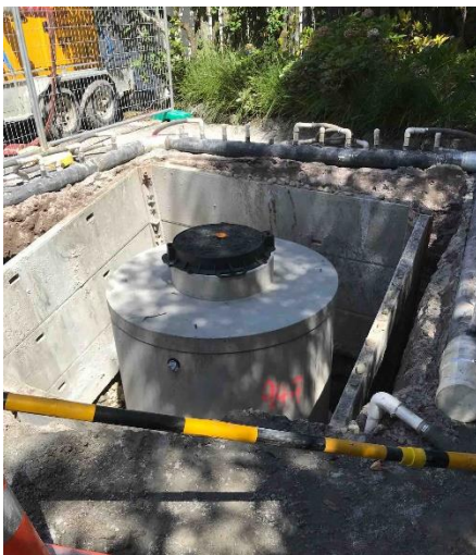
Trafficable concrete system installed at Hauparu Bay site. Dewatering equipment, trench shield and work area isolations in
