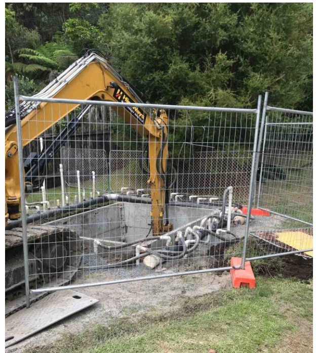
Haparua Bay site prepared for tank install. Dewatering equipment, trench shield and ground protection mats in place.
