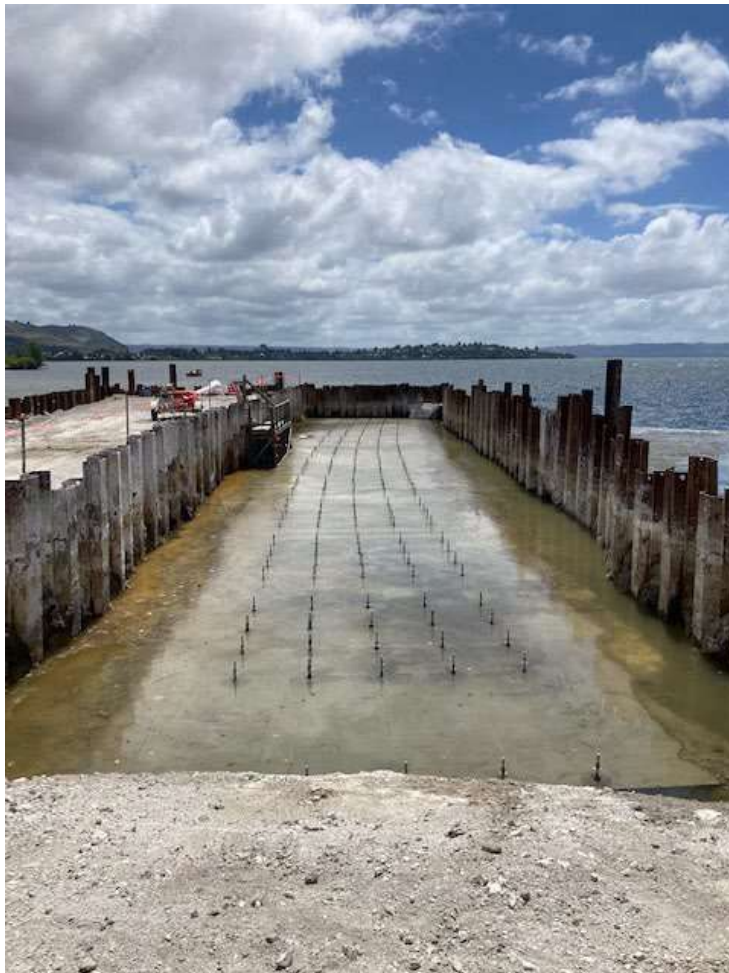
Above: Ground stabilisation and micro-piles prepared for the base of the western boardwalk in Stage 5
