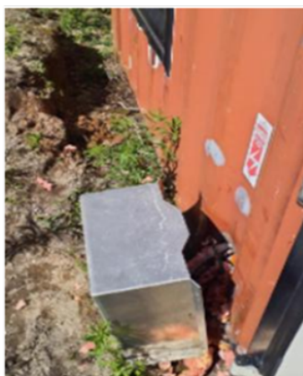
Pictured: Cable box torn off container
