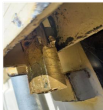
Pictured: Padlock badly damaged but still holding
