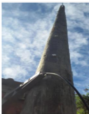
Pictured: Pole with coms wire stripped
