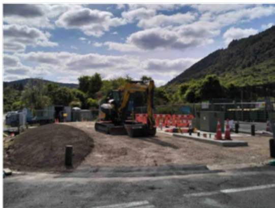
Pictured: Transfer Pumping Station
