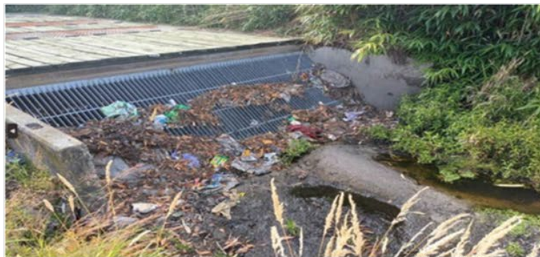
Above: Repaired gross pollutant trap working effectively to capture rubbish and debris after a rain event during the Christmas break.
