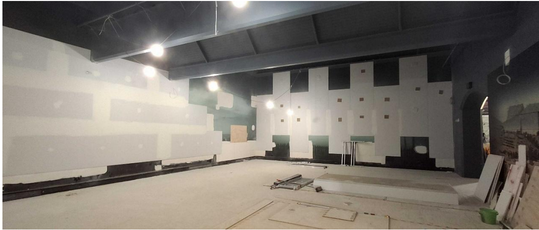
Figure 4: South Wing wall lining 30/10
