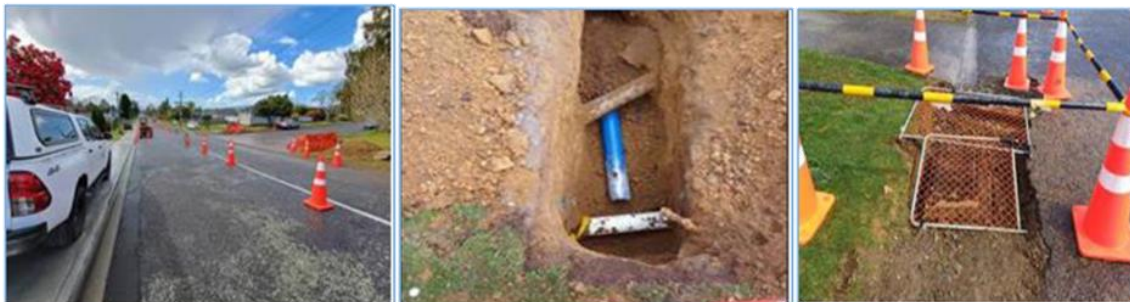
Photos above: Works began this week at the Otonga Road/Wychwood Crescent intersection to repair multiple stormwater main lines and cesspit leads, as well as the relocation of a water main that previously ran through the middle of a stormwater line. Priority has been placed on undertaking these repairs prior to an earmarked reseal of the road. Works are being undertaken by William's Drainage Ltd.
