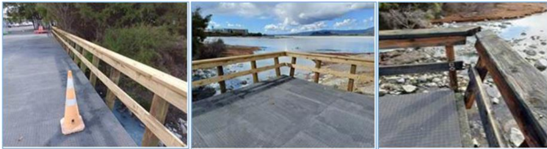
Photos above: Safety issues were noted with the old balustrade surrounding one of our gross pollutant traps which doubles as a viewing platform behind the Sudima Hotel. The old railing had a large amount of rotting timber and corroded fixings that had made the area unsafe. A like for like replacement balustrade was recently installed in a highly cost effective and timely manner by Edwards Fencing Ltd.
