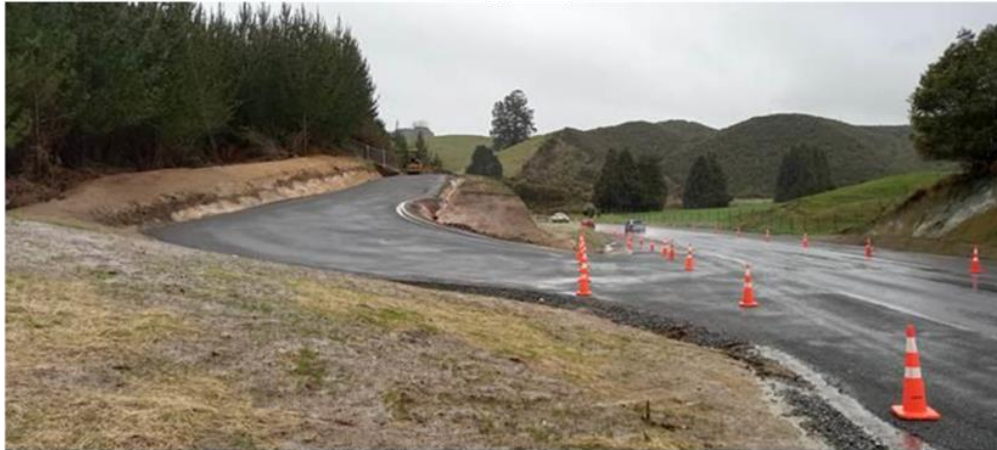
Above: New forest access point created for forestry operations off Tarawera Road
