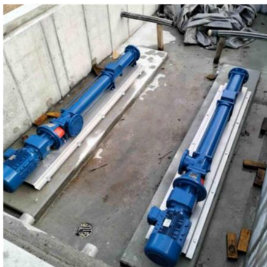
Photo above: Cliff Road Pumping Station
