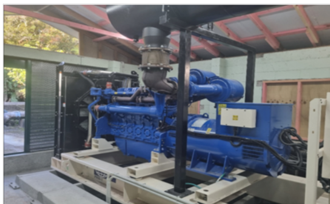
Photo: Generator at the Karamū Tākina (Central Urban) Water Treatment Plant
