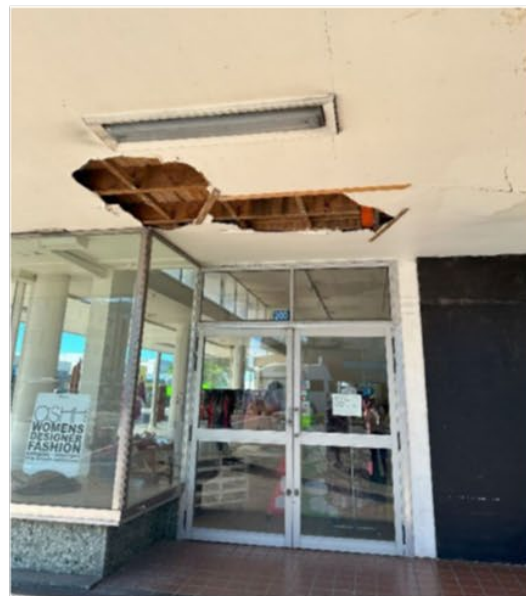
Main Street building decay. Gladstone Rd
