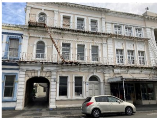
Masonic Hotel decaying façade. Lowe St
