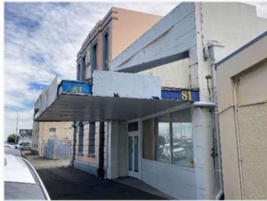
Deteriorating building. Childers Rd
